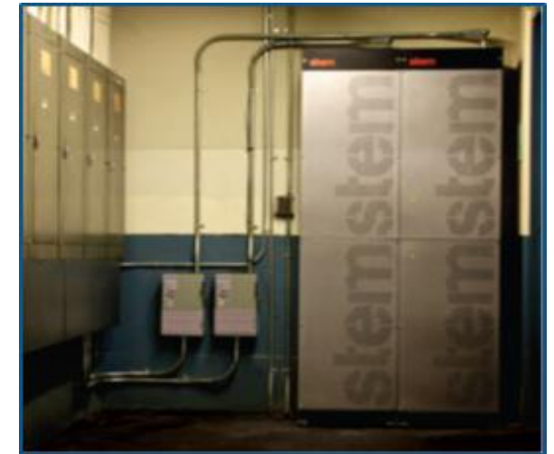
A commercial installation of Stem's PowerStore energy system.
