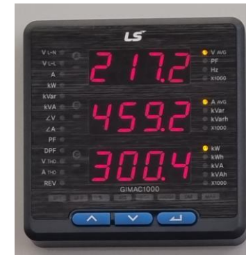
RLC Load Panel Meter [Vrms] [A_avg] [kW]
