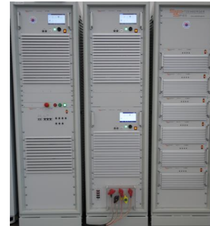
Power Amplifier (30kW)
