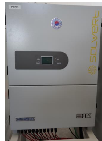
PV PCS (50kW)
