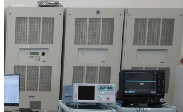
AC Source (270kW) Power Analyzer Oscilloscope
